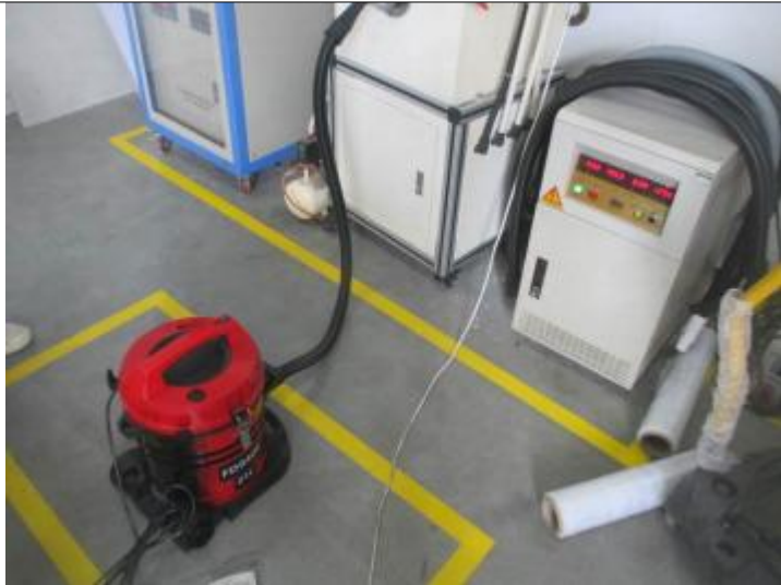
Low voltage starting check
