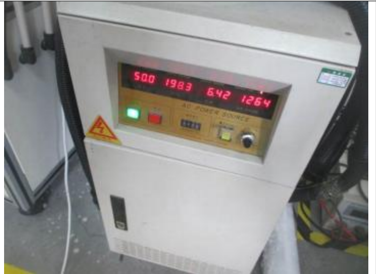
Low voltage starting check
